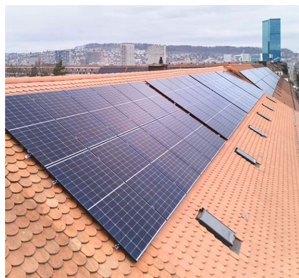
↑ PV-Anlage Hard West.
